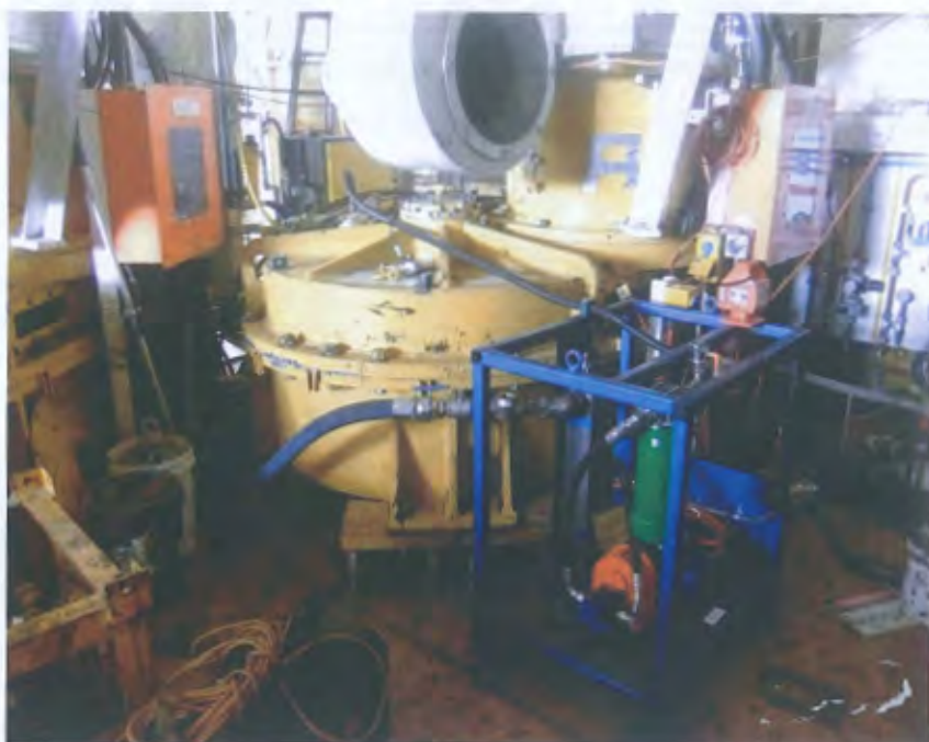
BHP kidney loop installed on gearbox.
